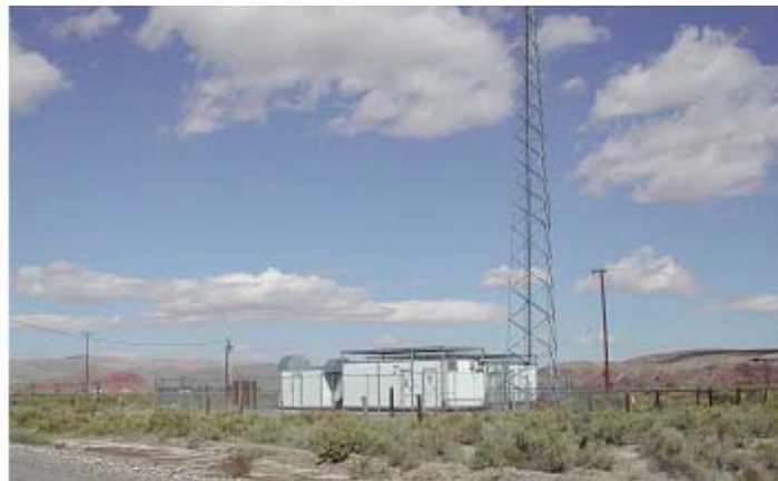
Tower near Carlin Connection to UPRR
